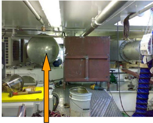
Figure 3.5: Urea tank in the aft ship.
