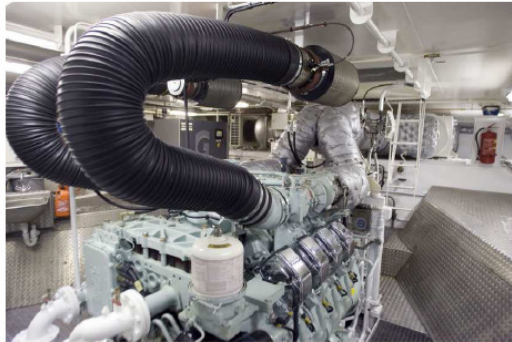
Figure 3.2: Main engine with complete installation.
