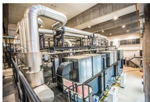
Heating plant Klagenfurt
