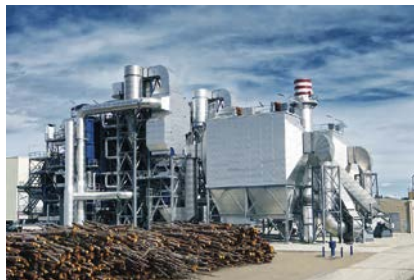
Flue gas cleaning, ESP/electrostatic precipitator
